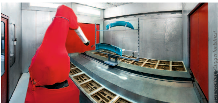
The filter boxes are also used for overspray filtration in the automotive supply industry
